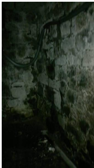
Figures 6 & 7: RHT 34 Possible arrow slit window and cellar wall, taken by Kirstin MacKintosh
